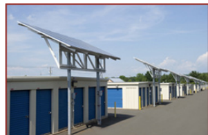
A PV system at Storage Investment Management's Newington facility, Planet Self Storage.
